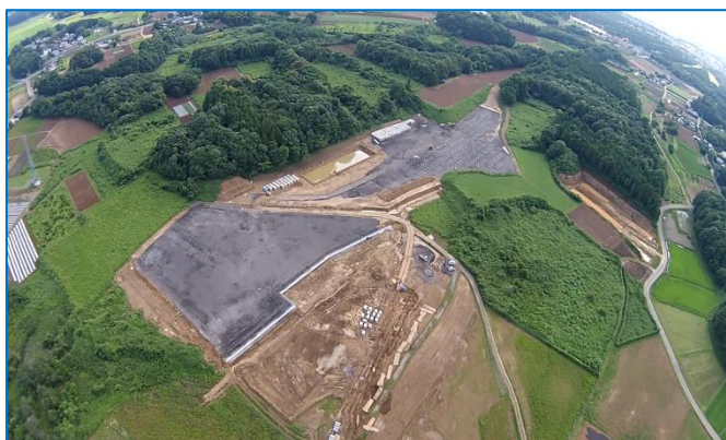
Aerial view of the 2 MW PV plant a few days ago
