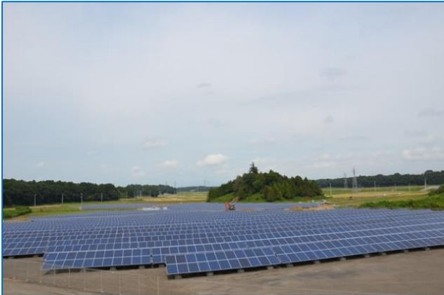
View of the 2 MW PV plant a few days before its commissioning
